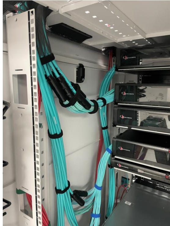
64F MTP Trunks & Lightverse between leaf & spine switches
