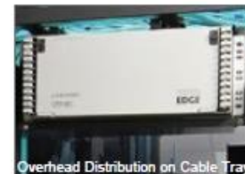
Overhead Distribution on Cable Trays
